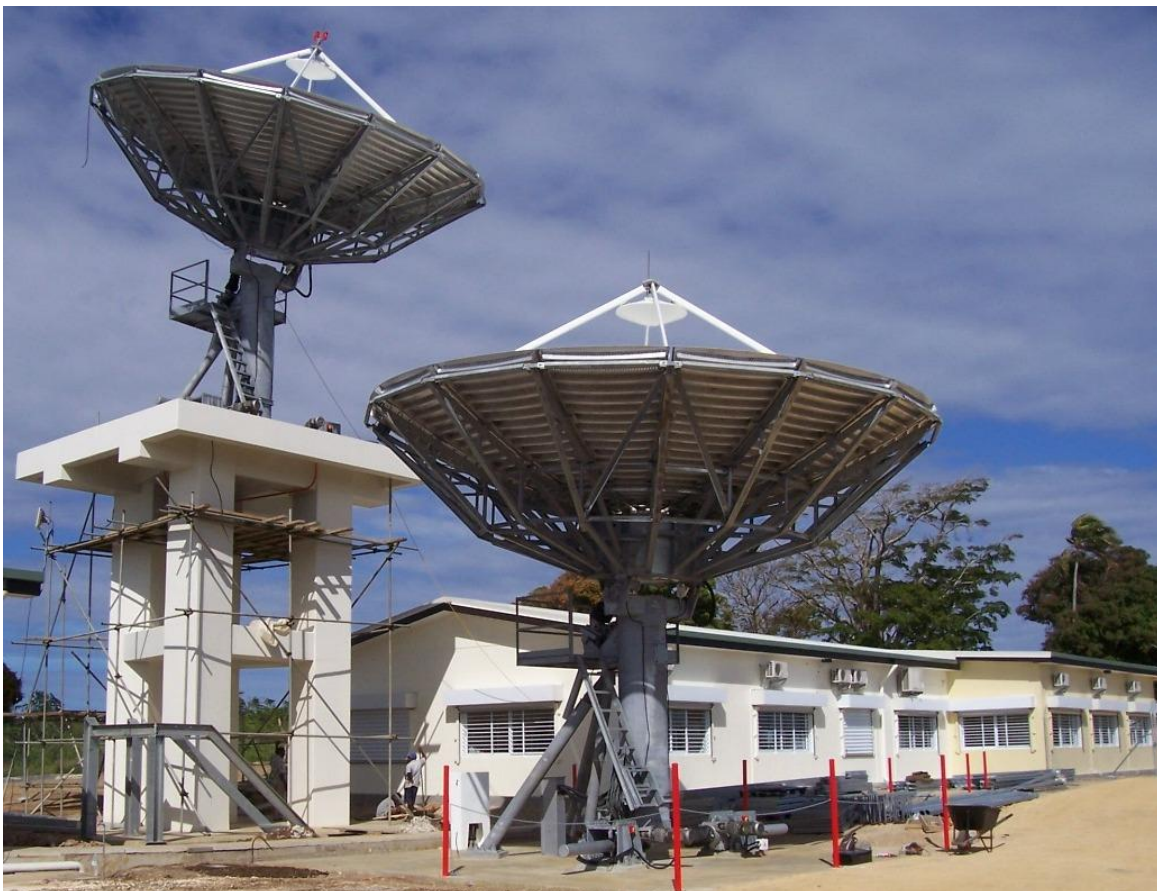
PDS Data Center Complex - Vanuatu
